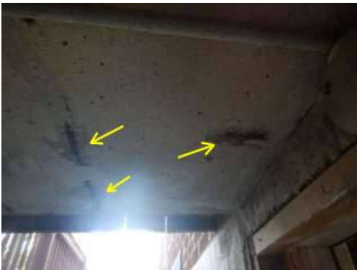
Photo 6-5 The ceiling over the basement stairwell has steel rebar rusting and needs to be sealed and maintained to prevent further damage.
