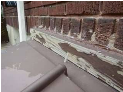
Photo 4-3 @ lintel over hatch
